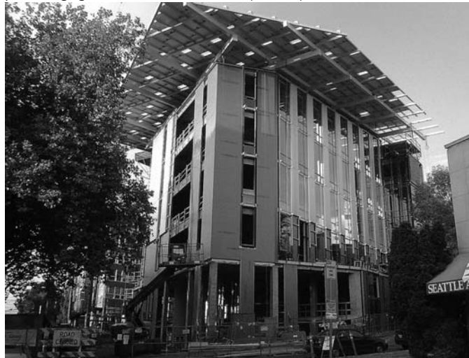
So far, 15 different projects, from New York State to Hawaii, have been certified as "Living Buildings." The likely 16th is Seattle's Bullitt Center (pictured here in progress), a six-story solar-powered "net zero" building designed to make extensive reuse of rainwater and day lighting and which features many other green amenities. Credit: Joe Wolf, courtesy Flickr
